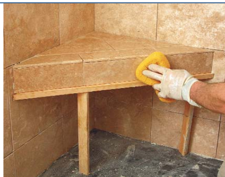
After the mud is prepped with successive layers of thinset, waterproof membrane, and thinset, tile is laid across the top, then the front. Temporary braces keep the edge tile in place until the thinset bonds.
