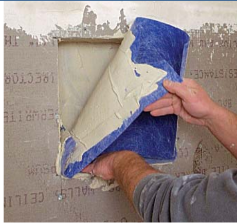
After coating the recess with thinset, cover the inside with a piece of waterproof membrane, folding and sealing corners as needed. Prefab inserts are also available.
