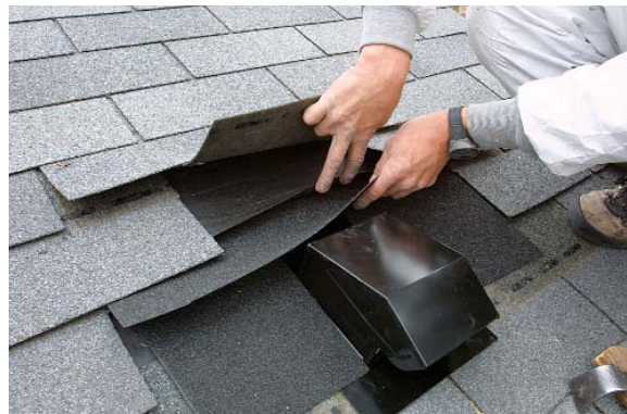
Sides first. Slipped below the underlying tar paper and overlapping the flange, the flashing extends onto the shingle below.
