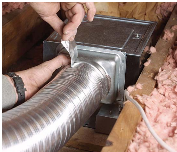
Seal all ductwork tightly. The duct is slipped all the way onto the fan's exhaust port and sealed airtight with aluminum duct tape. Don't use common fabric-backed duct tape, which will deteriorate with time.
