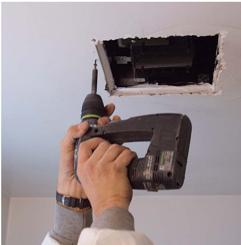
Screw through the ceiling. Drywall screws anchor the fan to the ceiling and will be hidden by the fan's cover and light.
