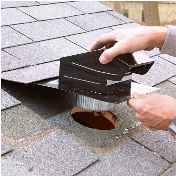
The vent faces down the roof. Slip the vent into the hole with the opening facing down, and secure it at each corner with galvanized roofing nails.
