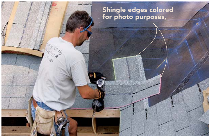
The first course is always a weave. For every valley variation, except the open metal valley, the first course is a weave. The shingle from the larger roof plane overlaps the shingle from the smaller plane.
