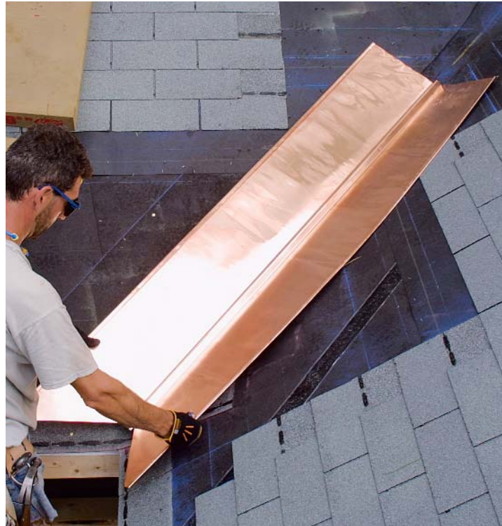
An extra crimp for extra protection. An inverted V in the center of the valley liner helps to channel water down the valley while allowing for expansion and contraction widthwise.
