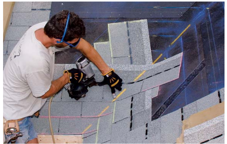
A handy nailing gauge. Nails always should be kept at least 6 in., or the distance between an outstretched thumb and index finger, away from the center of the valley.
