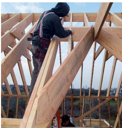
Just as if it grew here. When the valley is in place, the 72° heel cut lies flat against the doubled common rafters. The rafter bottoms are kept flush, and the dormer roof sheathing hides the height difference in the rafters.
