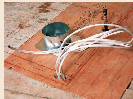
1. Pull wiring after rigid materials. The plywood subfloor was put in place after the duct was installed and the gas line was checked for leaks.
