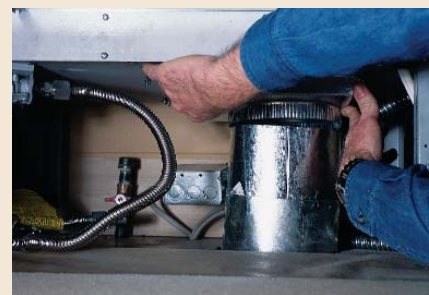
3. Accurate layout leads to easy tie-ins. The duct, gas and electrical connect easily and are accessible for maintenance.
