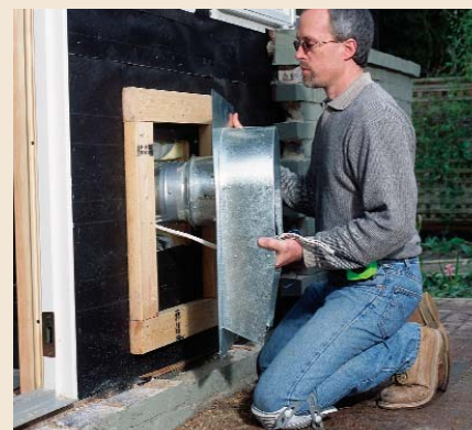
2. Assemble the remote blower before installation. Screws and duct tape join the assembly before installation. A 1/4-in. space (for easy future removal) around the blower's perimeter was later weatherproofed with exterior caulking.
