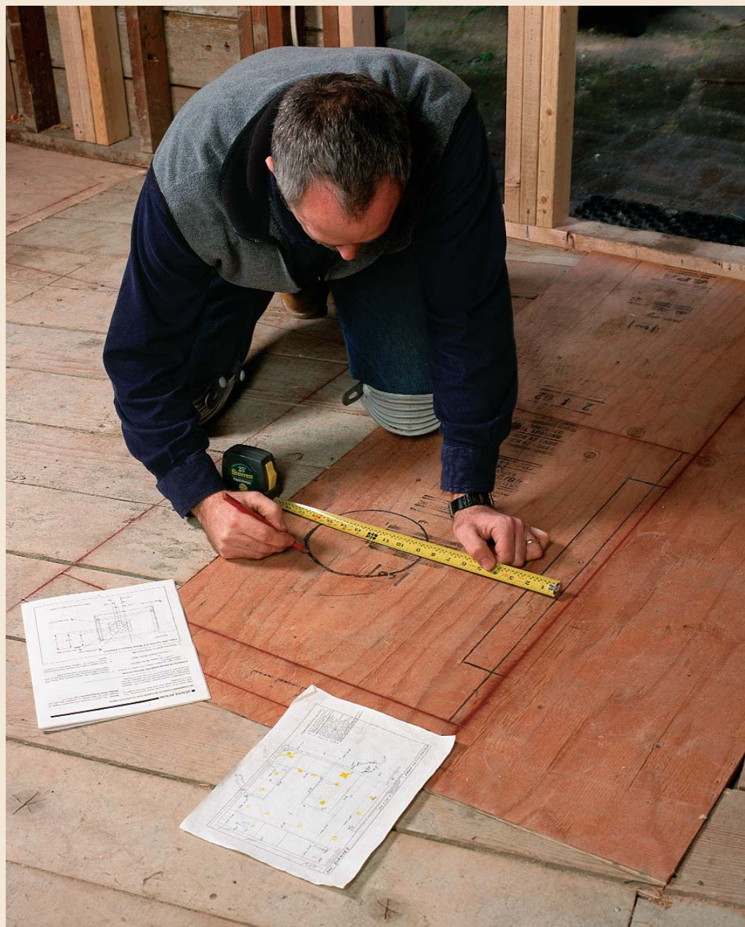
The range location is drawn on a new plywood subfloor. Using the manufacturer's installation instructions, the author determines the exact locations of the duct, gas pipe and wiring.
