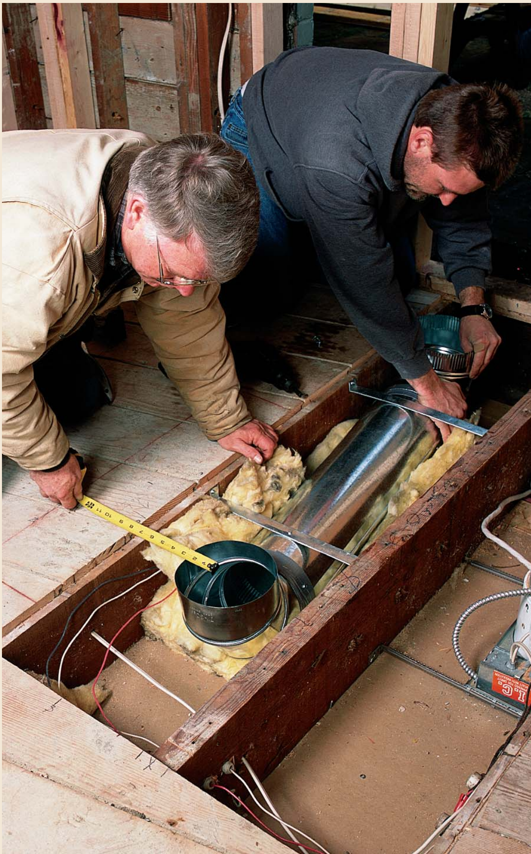
With the plywood removed, the assembled duct is set in place. Measurements taken from the subfloor edge verify the duct's location. Insulation below dampens the noise, and sheet-metal straps hold the duct fast.
