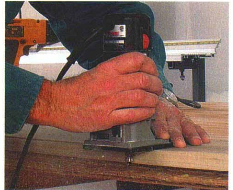
A quick pass with a flush-trimming router evens up the edges. Most of the glue squeeze out had been scraped off to avoid fouling the bit's bearing.
