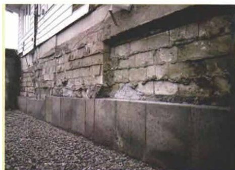
A single-face wall keeps the soil where it belongs. Excavation for the full basement addition left soil exposed below the existing foundation. The concrete wall poured against the soil keeps the foundation from being undermined.
