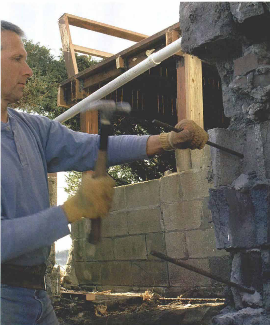
Connecting the old with the new. Rebar driven into drilled holes every 18 in. ties the addition foundation to the old foundation.
