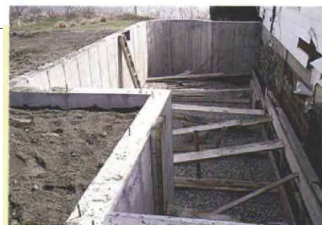
You can't have too much bracing. To resist the pressure of wet concrete, the forms are braced every few feet top and bottom, with the addition walls providing a strong backer for the braces.
