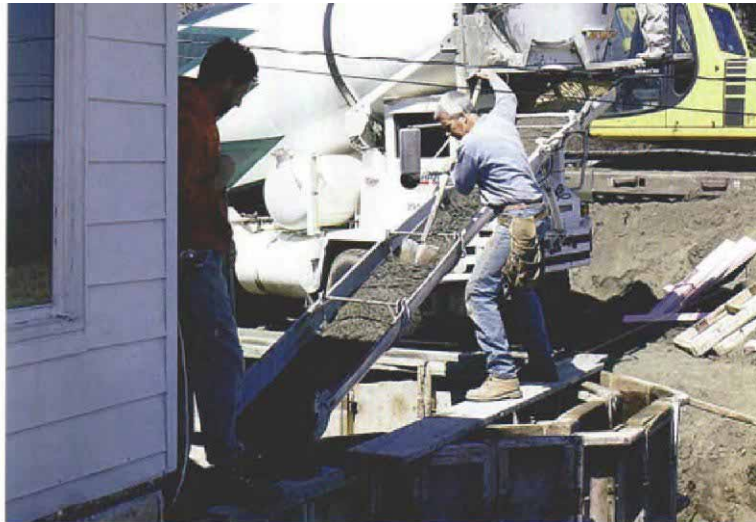
A stiff mix starts the pour. The pour starts at the existing foundation, and a stiff mix helps to plug any small voids where the forms meet the old foundation.
