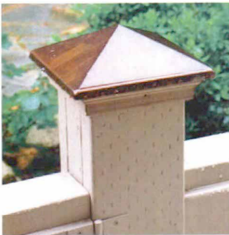
Quick fix for a bad problem. To protect vulnerable end grain, the author covers the tops of 4x4 posts with ready-made copper caps.
