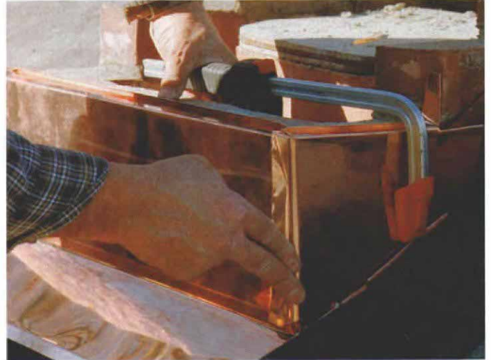
Wrapping the corner. For appearance's sake, the author trims the bottom of the first corner piece to match the roofline and carefully wraps the front corner. To make sure that water never finds an entry point, he cuts the back leg 1 1/2 in. long and folds the top lip up the face of the brick.
