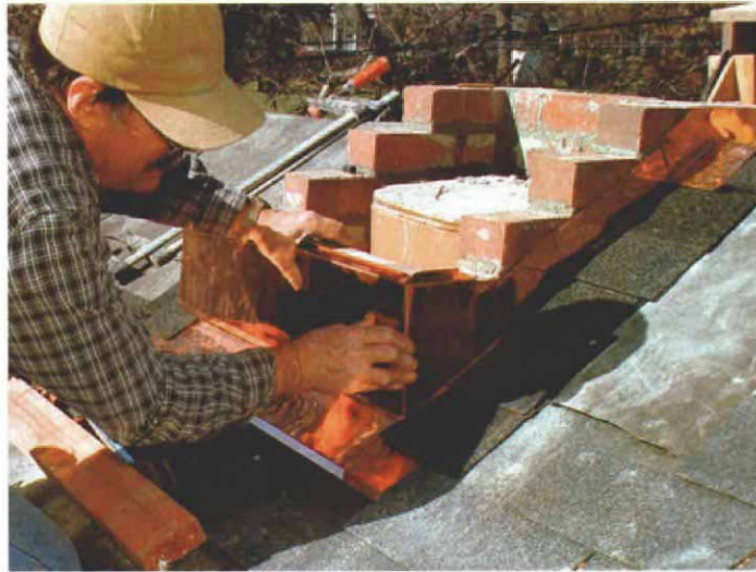
Placing the counterflashing. After bending the sides to match the profile of the chimney, the author slips the counterflashing over the bricks and temporarily secures it with a clamp. Note how the bottom of the side piece is cut to follow the pitch of the roof.
