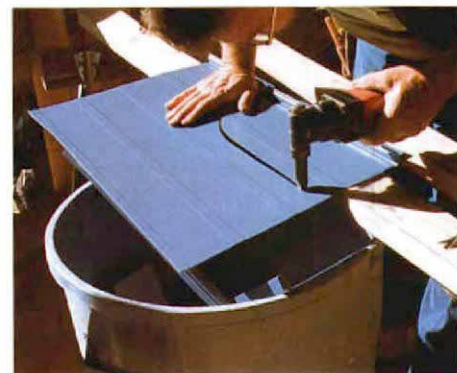
Munching metal. A tool called a nibbler can cut just about any shape in a metal-roofing panel, but the shavings are messy.
