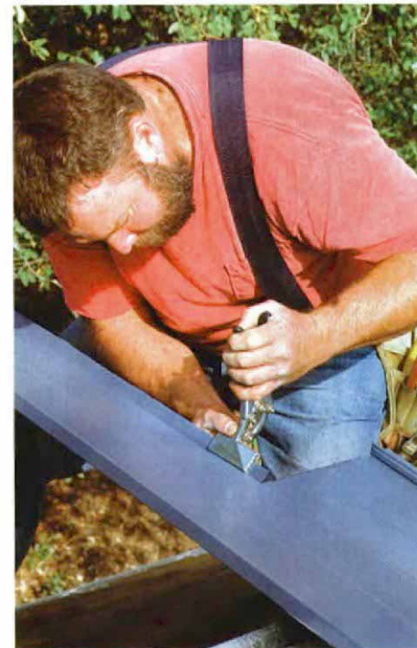
Special pliers help to bend the roofing. To make a rib for the edge of a roofing section, special pliers called hand seamers bend the edge in gradual increments.
