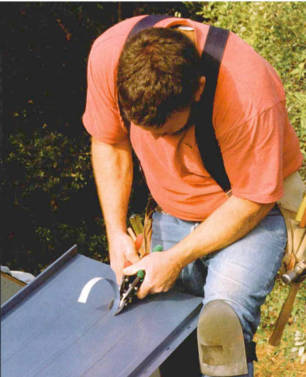
Dueling snips. To cut straight lines in a roofing panel, right-handed and left-handed snips are used side by side, and the waste curls up harmlessly in between.
