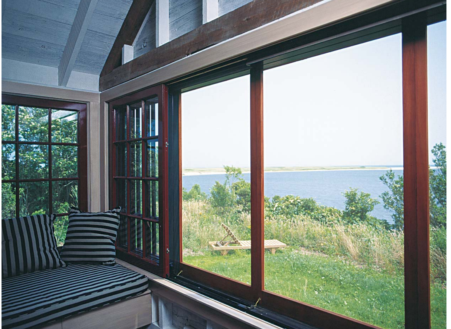
Ventilation and storm protection in one. A pair of telescoping windows span a 21-ft. width on the ocean-facing east wall of the cottage. They can be closed quickly in bad weather. Photo taken at F on floor plan.
