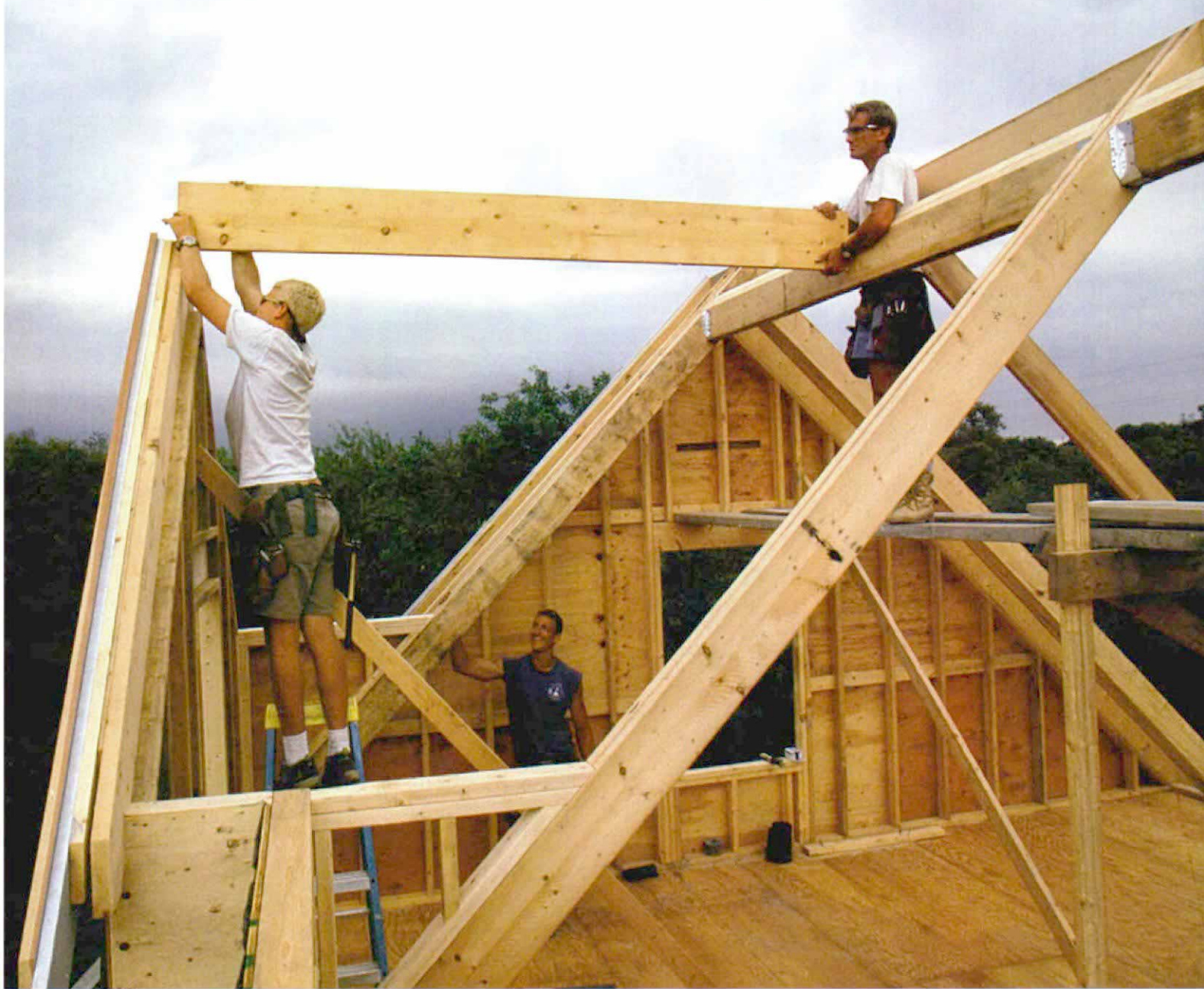
Doghouse ridge drops in. The doghouse ridge connects the outer wall of the doghouse dormer to the header.
