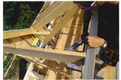
Corner of the valley. Angles that are taken on each side of the string determine the corner cuts that are needed for the ends of the valley rafter.
