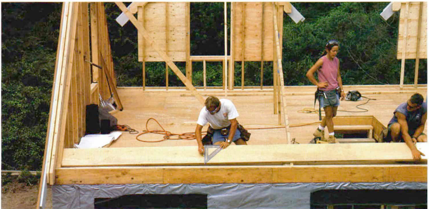
Laying out the ridge. To get the rafter layout to match precisely, the layout on the plates is transferred directly to the ridge stock.
