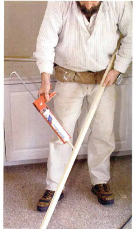
Face frames are glued to the walls. To help stabilize the sides of the shelf sections, the face-frame edges are coated with construction adhesive before being nailed to the shelf sides.
