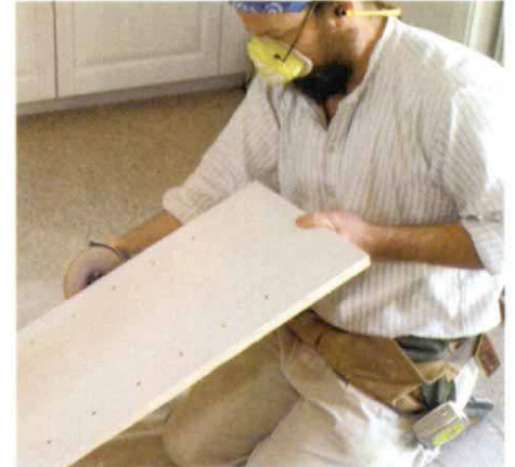
Grinding to the line. An electric grinder creates a bit of dust, but the grinder is easy to control and allows a feather edge to the scribe line.
