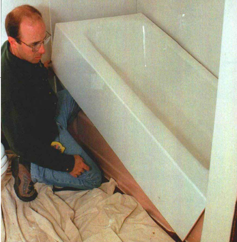
Acrylic is lightweight and easy to maneuver. Connecticut contractor Paul Foley fits a new acrylic tub over a cast-iron fixture that will remain in place. The two are bonded with silicone caulk and butyl tape.
