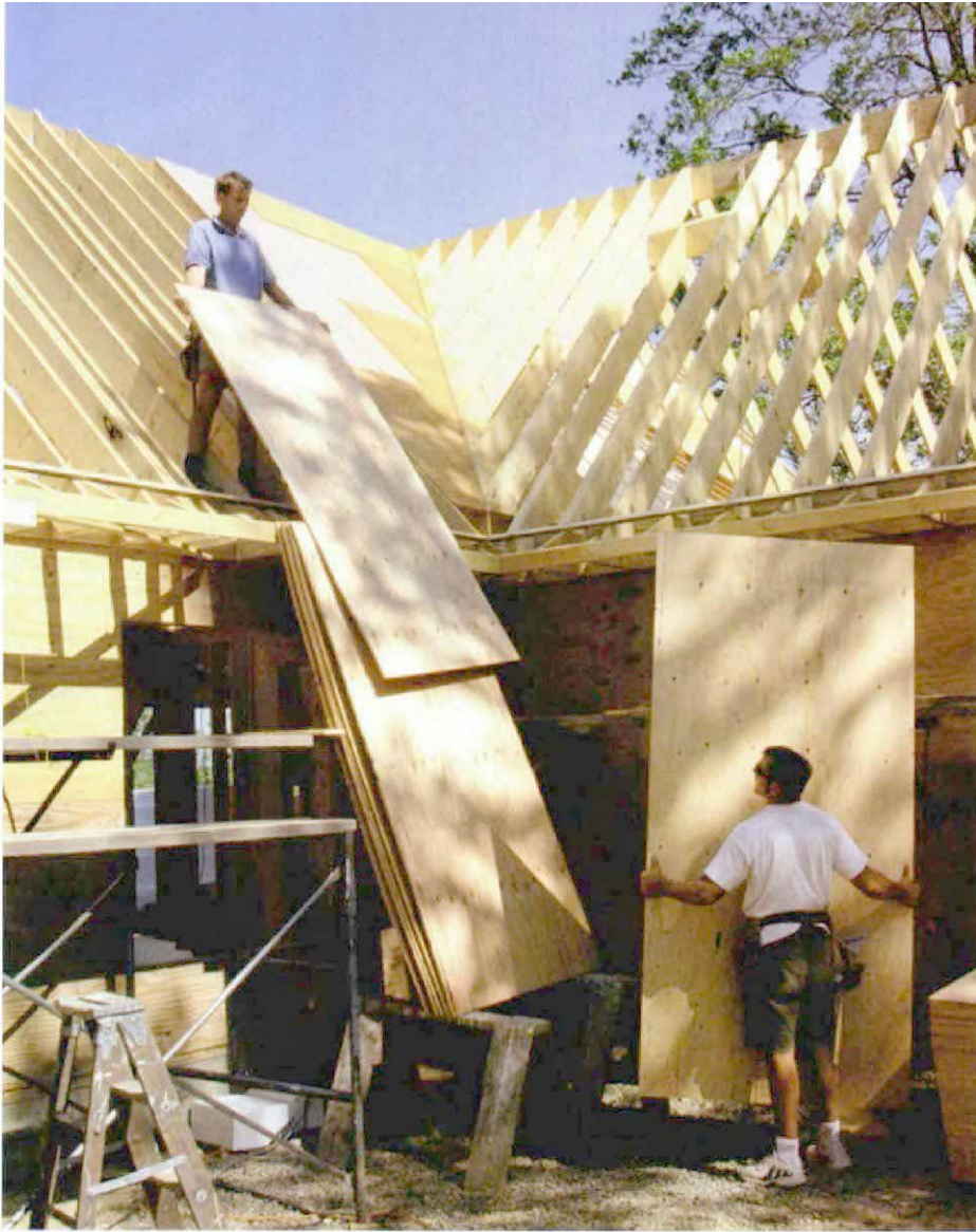
Sawhorses make for easy picking. The easiest way to get the sheathing onto the roof of a single-story house is to lean the sheets against the fascia on top of two sawhorses.
