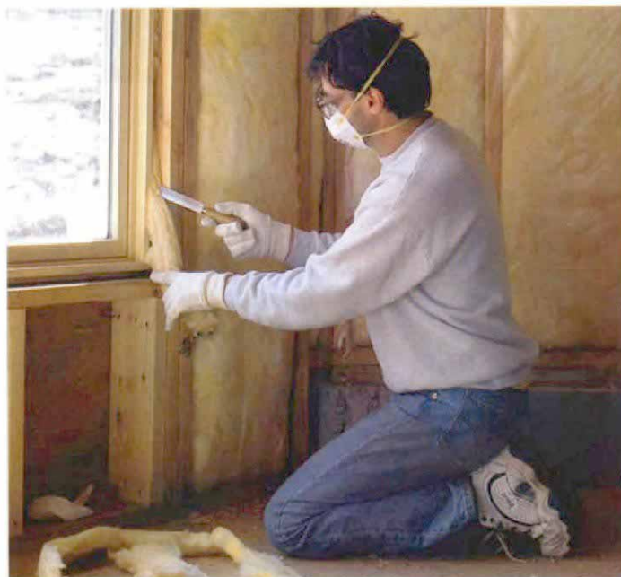
Insulating around windows requires the right amount of fiberglass. Too much fiberglass packed next to a window jamb cannot insulate properly and distorts the jamb, making the sash bind. The fiberglass should be able to expand and fill the space.
