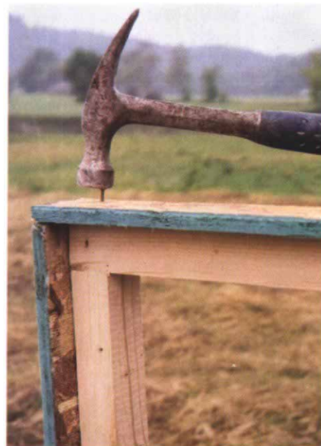
Simple wooden form creates a stronger cap. The author nails a frame of 2x lumber together for the basic form. Strips of OSB nailed to the sides give the form a depth of 1 in.
