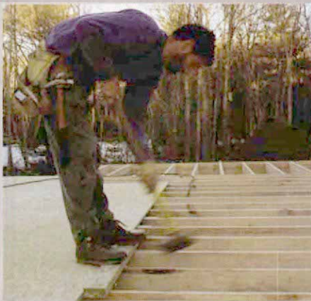
A sledgehammer snugs the sheathing into place. A 2x block protects the grooves in the edges of the sheathing as it is tapped into place with a sledgehammer.
