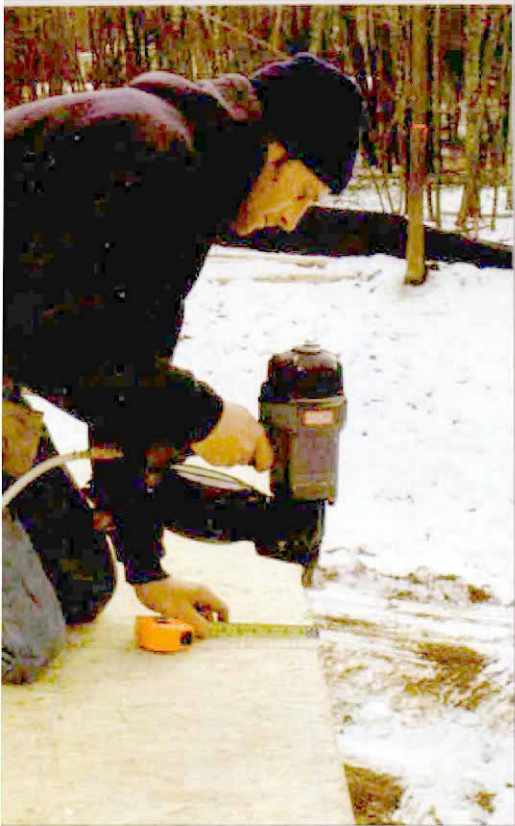
Straightening the final edge. When all the sheathing has been installed, a line is snapped 1½ in. from the ends. The rim joist is then moved in or out until it lines up with the end of the tape.
