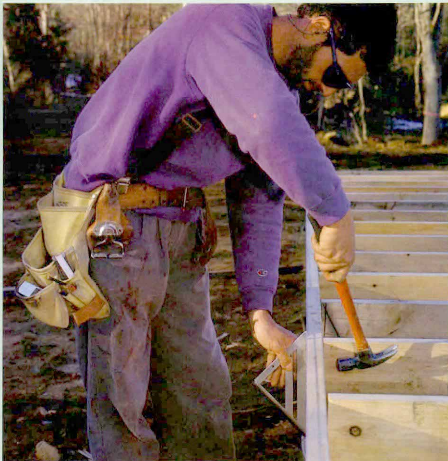
Tweaking the rim joist. Before the sheathing goes on, a string is run along the top edge of all the rims that run perpendicular to the joists. The rim is tapped in or out and checked with a square until it is perfectly straight.
