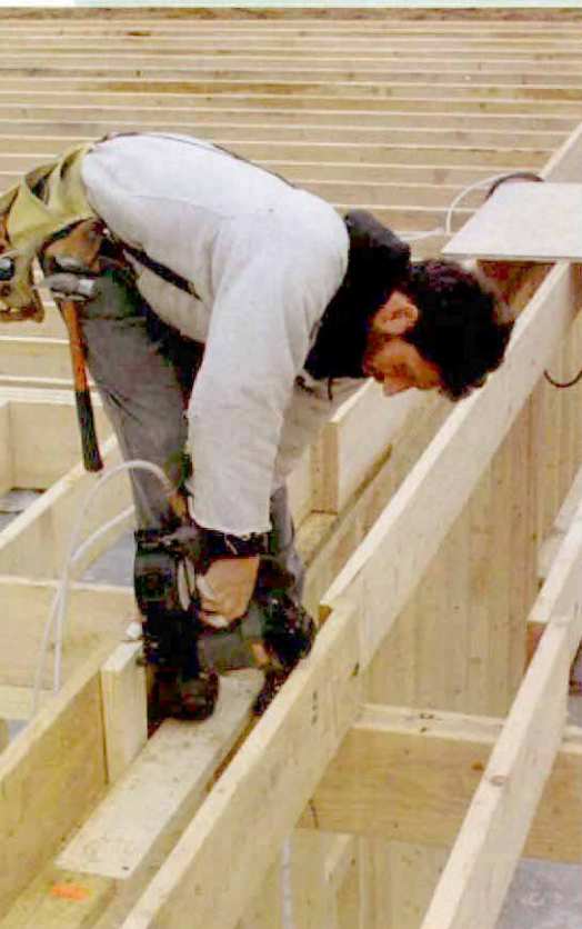
Squash blocks carry loads from above. Two-by blocks called squash blocks cut slightly longer than the height of the joist help to transfer loads directly to the sill plate or carrying beam. Here, the squash blocks are installed under header-bearing jacks for a sliding door above.
