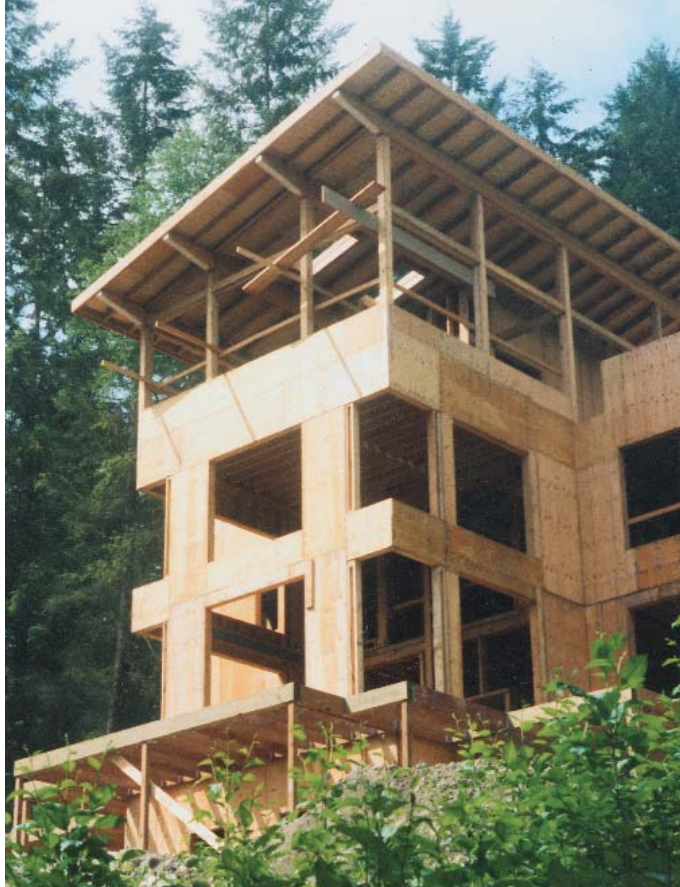
A patchwork of small shear panels. Nearly every exterior surface shown in this construction photograph is a shear panel of \frac{3}{8} -in. plywood over 2x6 framing. Already framed in is the horizontal steel wind beam, which wraps around the two-story space shown here between the first and second floors.
