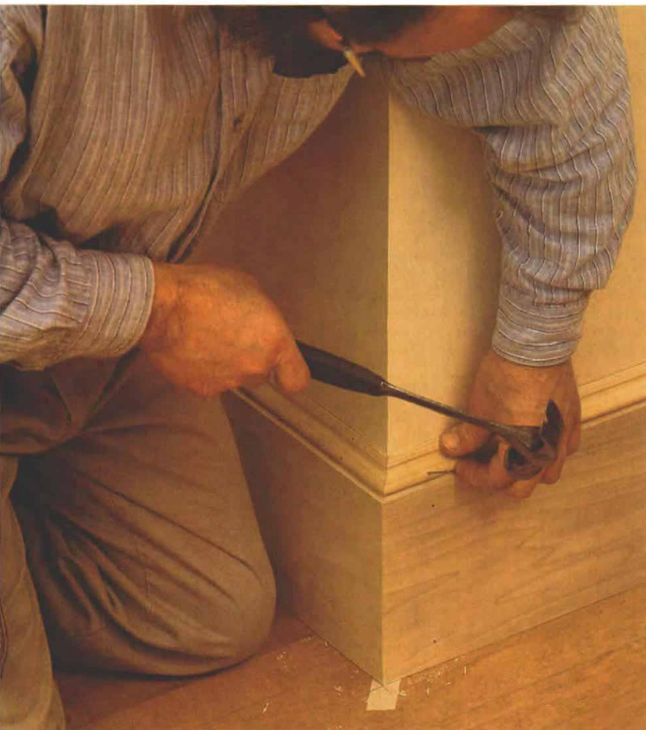
Base cap is nailed on last. Besides adding a decorative profile, the base cap conforms to irregularities and hides any gaps between the wall and the baseboard. The cap can be nailed either to the wall studs or to the baseboard.
