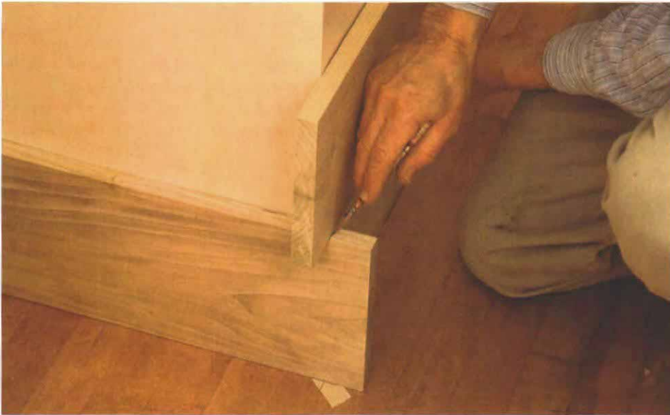
Mark baseboard in place when outside corners aren't square. Pencil lines on a piece of tape show where the baseboards intersect at the floor. A line connecting this point with the point of intersection at the top of the baseboard (being marked here) establishes the outside edge of the miter. Similar lines on the back of the baseboard determine the bevel angle.
