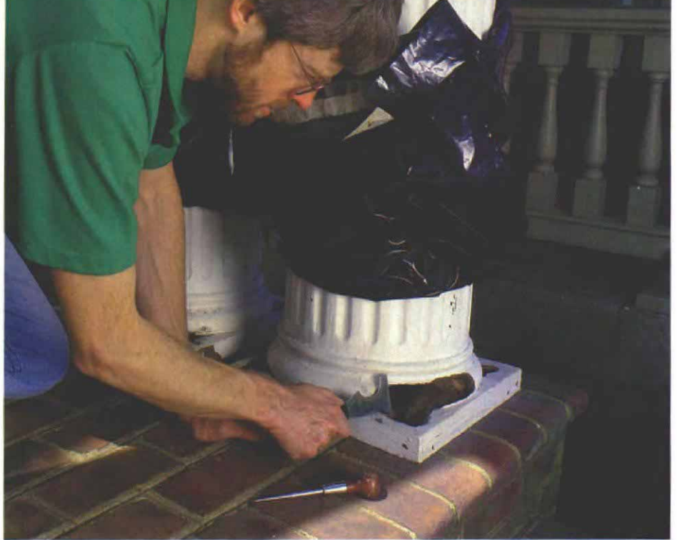
Getting down to sound wood. The first step is removing loose, crumbly wood. A five-in-one painter's tool and an awl are best for digging out any wood that is not still firmly attached.
