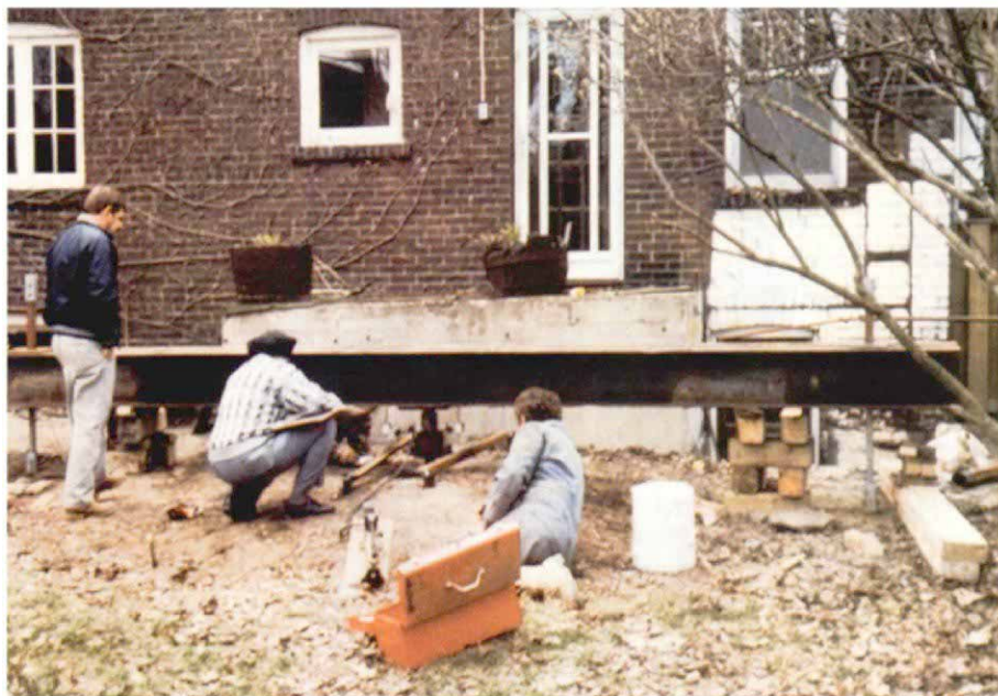
Piers were tested on site. In a test required by the Toronto building department to rate the strength of helical piers, three piers were driven into the ground 7 ft. o. c. A steel I-beam was bolted to the two outside piers, and a jack was placed between the center pier and the beam. The piers withstood pressure from the jack, and the city issued a building permit.
