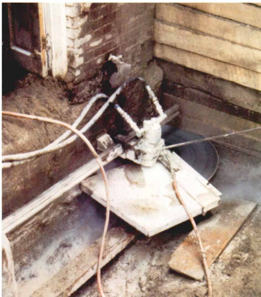
Separating a house from its foundation. A large concrete saw was used to cut the foundation walls free from the house. The walls had been sinking into soft soil and were too deep to support from below. Above the cut, the house was raised by a series of helical piers.
