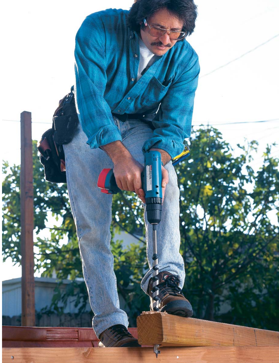
Twelve-volt drills with 1/2-in. chucks can drive bigger drill bits. A large, self-feeding auger bit is no problem for most 12v drills in low gear, making them attractive to other tradesmen such as plumbers and electricians.
