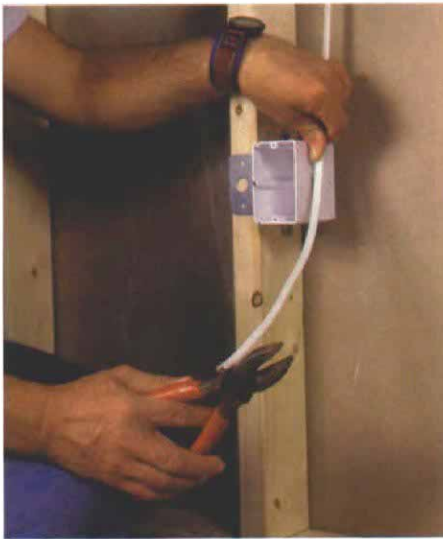
Leave plenty of slack. Run the cable about a foot past the box to give yourself plenty of wire to make splices and connections.
