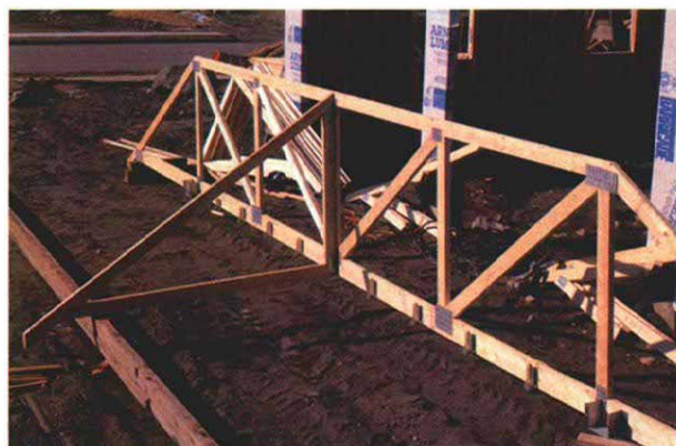
A jack truss holds the girder truss upright. The center face jack truss is tacked to the girder truss to keep it vertical while the rest of the face jacks are installed.
