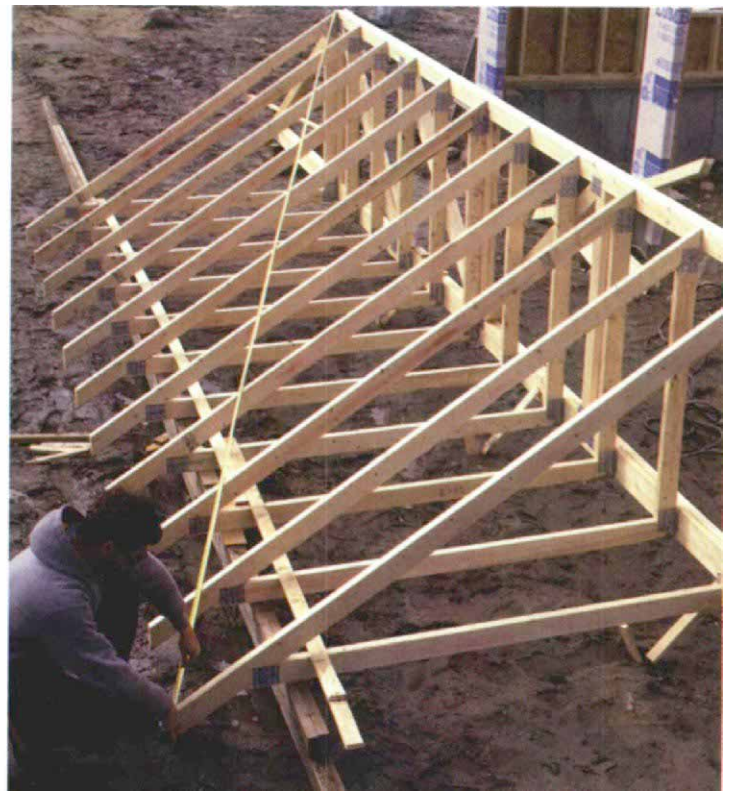
Diagonal measurements square the system. Measurements are taken between the two outermost jack trusses, and the tails of the trusses are moved in unison until the measurements are equal.
