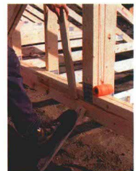
Straightening the girder trusses. A temporary brace keeps the girder trusses straight while they are being nailed together.
