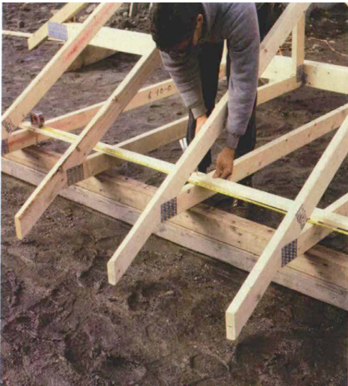
A furring-strip spacer keeps the tails in place. Before the system can be squared, the tails of the face jack trusses are spaced according to the layout and held in position with a piece of 1x3.
