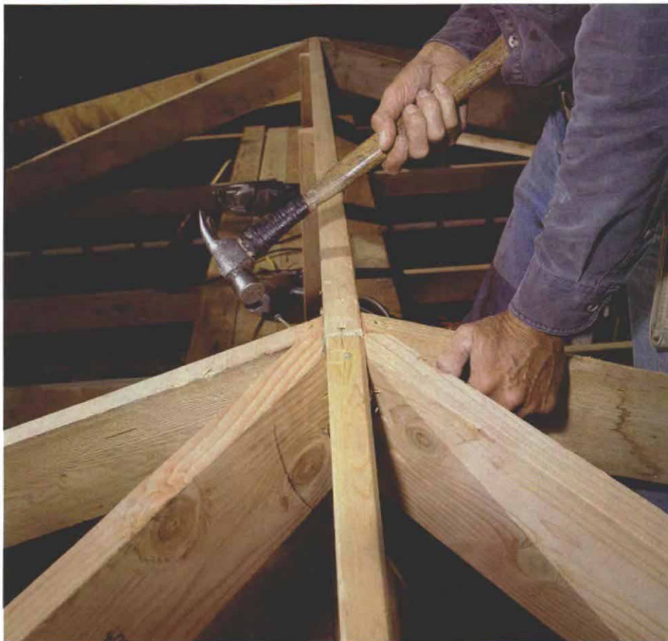
The hips and king commons come together at the ridge. The end of the ridge is the meeting point for all of the major framing members of the hip roof. After the end king common is nailed in, the hip rafters are installed, and the ends of the side king commons are nailed in next to the hips.
