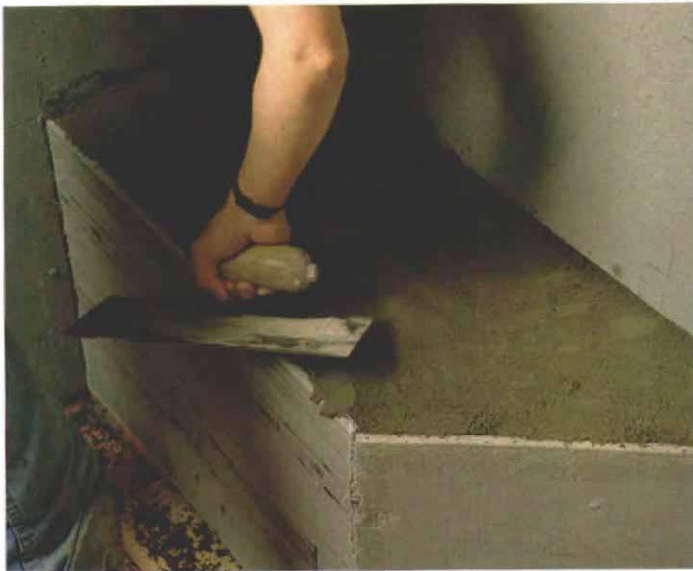
The marble for the seat goes on top of cement. The backerboard around the shower seat was left 1½ in. high, and then the resulting cavity was filled with cement, making the seat top virtually waterproof. A marble slab was used for the seat to eliminate grout joints.
