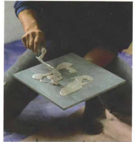
Epoxy seals the backs of the green-marble tiles. Green marble reacts badly to water-based adhesives, so the backs of the tiles are sealed with nonporous epoxy. A trowel spreads the thick and gooey epoxy.
