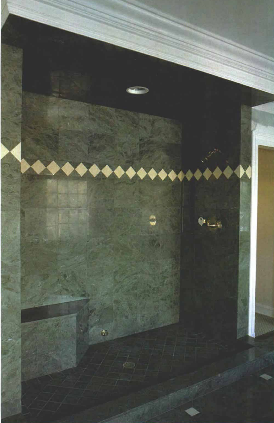
A showy shower out of stone. Before installation, marble tiles are arranged so that the veins and colorations all work together. The tiles are put on as flat as possible and tight to one another to give the impression of a solid slab of marble.
