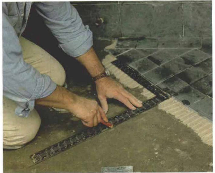
Tiling is tough on tools. A framing square is used to check the alignment of the floor tiles and to keep them running straight. But it's hard to do without plunking the tool down in fresh adhesive, which isn't great for the square.
