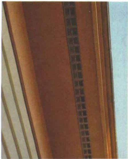
Continuous vents keep roof washed in cold air. A ridge vent draws cold air from the continuous soffit vents uniformly across the underside of the roof sheathing.
