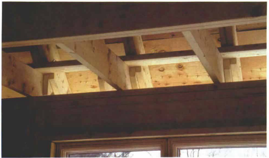
Elevated rafters make room for insulation. The builder made room for a thick blanket of insulation above the exterior wall by nailing the heels of these rafters to a toe board that sits on top of the ceiling joists. This construction method also maintains an adequate ventilation space between the sheathing and the insulation so that air can flow from the soffit vent to the ridge vent.
