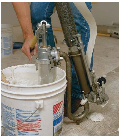
Tape faster with the automatic taper. Drywall taping gets done quickly with an automatic taper (top photo). A pump (above) is used to fill the automatic taper with compound.
