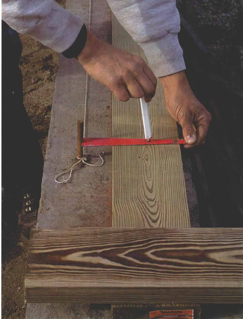
A simple jig locates the bolt holes. With the sill stock lined up on the inside of the chalkline, a jig with a U-shaped end is held against the bolt. The bolt-hole location is marked through a hole 5\frac{1}{8} in. from the U.
