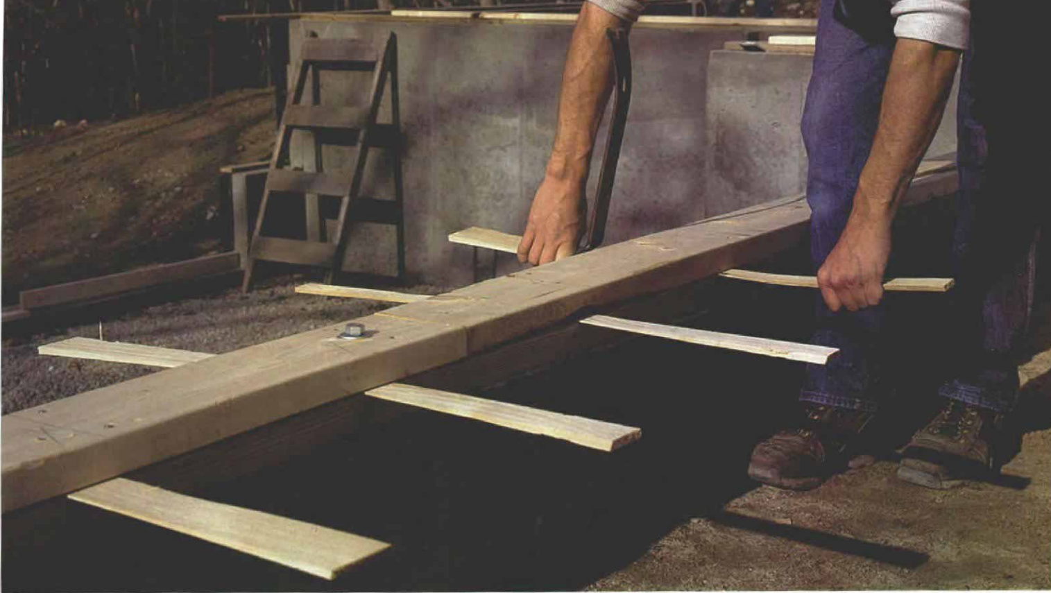
Shims correct an out-of-level foundation wall. If there are dips in the foundation, the two sills are pried apart with a flat bar. The nails used to tack the upper sill in place now serve to hold the two sills apart while shims are inserted beneath the future joist layout.
