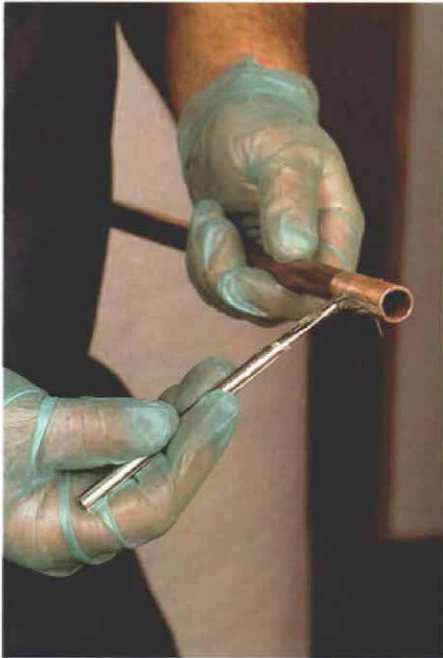
Apply an even coat of flux to the pipe. An acid brush full of flux is held against the pipe while the pipe is rotated to deliver a thin, even coat. Gloves protect the plumber's hands.
