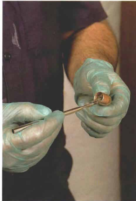
Don't forget to apply flux to the fitting. It is important to apply flux to the fitting as well as to the pipe before soldering. Flux cleans the copper when heated and prevents oxidation.
