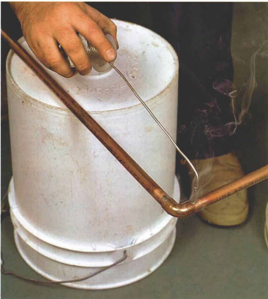
Solder melts and flows into the joint. After the pipe and fitting are assembled and heated, the flame is removed, and the solder melts into the heated joint.
