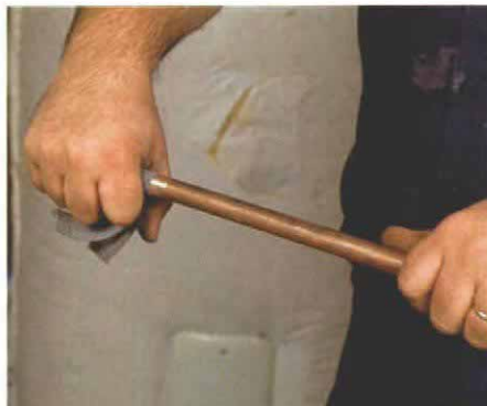
Plumber's sand cloth polishes the end of the pipe. To ensure a good bond for the solder, the ends of the pipe are polished with a short length of sand cloth that is rotated on the pipe until the pipe shines.
