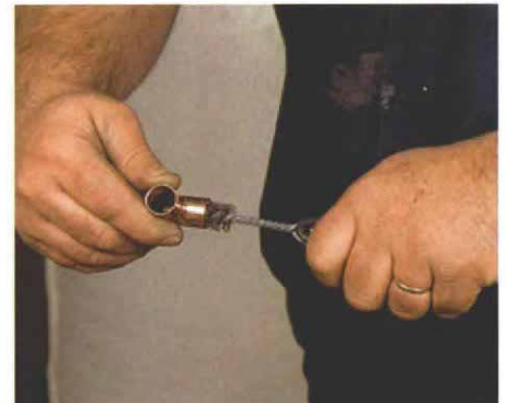
A round wire brush polishes the inside of the fitting. A wire brush that matches the diameter of the pipe is inserted in the fitting and twisted to polish the inside of the fitting all the way to the bottom.
