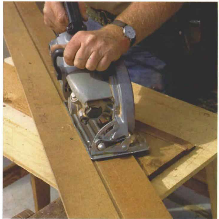
Shooting board for acute angles. A straightedge screwed to a pair of fences guides a circular saw through repetitive cuts that are beyond the swing of the sliding compound saw.
