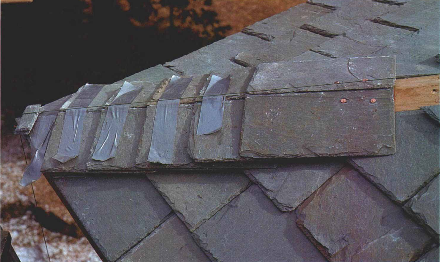
Duct tape and string help to align the saddle caps. The pieces of the ridge cap or hip cap (shown here) are bedded in silicone and fastened with two nails each into the wood strips the author attaches to all hips and ridges. To keep the caps straight, he sights along a string that runs from the eaves to the peak. Strips of duct tape hold the two pieces of the caps together while the silicone dries.
