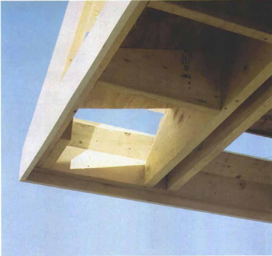
Tapered blocking frames the pediment cornice. This attractive detail on the gable begins with tapered 2x blocks that are installed between the last ceiling joist and the rough fascia of the pediment. The blocking forms the pitched roof above the pediment cornice, and it provides sound nailing for the roof sheathing.
