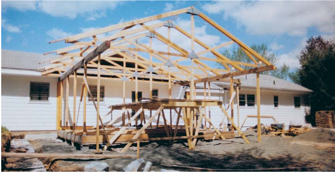
Scaffold provides work station for assembling trusses on site. Heavy 6x8 beams spanning from the house to the porch's corner posts carry trusses constructed of 2x4s and custom-made steel plates. Heavy beams allow for open walls that are sheltered by 2-ft. deep eave overhangs.
