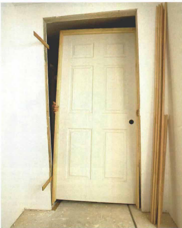
6. Don't forget the shim on the floor. Elevate the hinge jamb by placing it atop the butt end of a shim shingle as the door is lifted into position.
