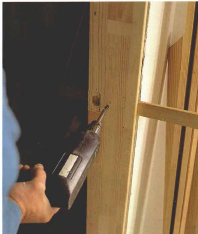
11. Reinforce the strike plate. After pulling the doorstop, run a screw through the strike jamb next to the door latch.
