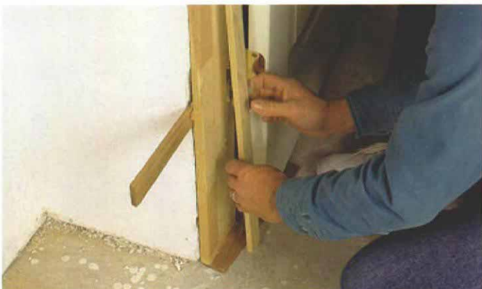
9. Remove the stops. Pry the doorstops from the bottom up. Then locate the screws that secure the jamb to the trimmer under the stop.
