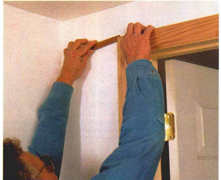
17. Shim problem casings at the corners. If the casings are out of plane, slip a shim under the corner so that both pieces bear on it. Then trim the shim flush with the casing with a utility knife.
