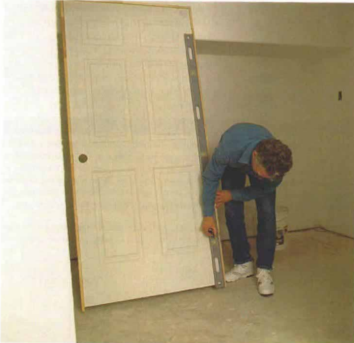
4. Note the hinge positions. Using a 6-ft. level as a story pole, the author marks the centers of the top and bottom hinges.
