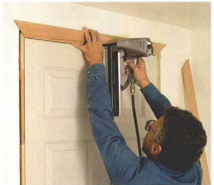
13. Casing starts at the top. Britton begins trimming a door by installing the head casing first. He affixes the casing with pairs of nails on 16-in. centers. One nail goes into the jamb, and another into the header.
