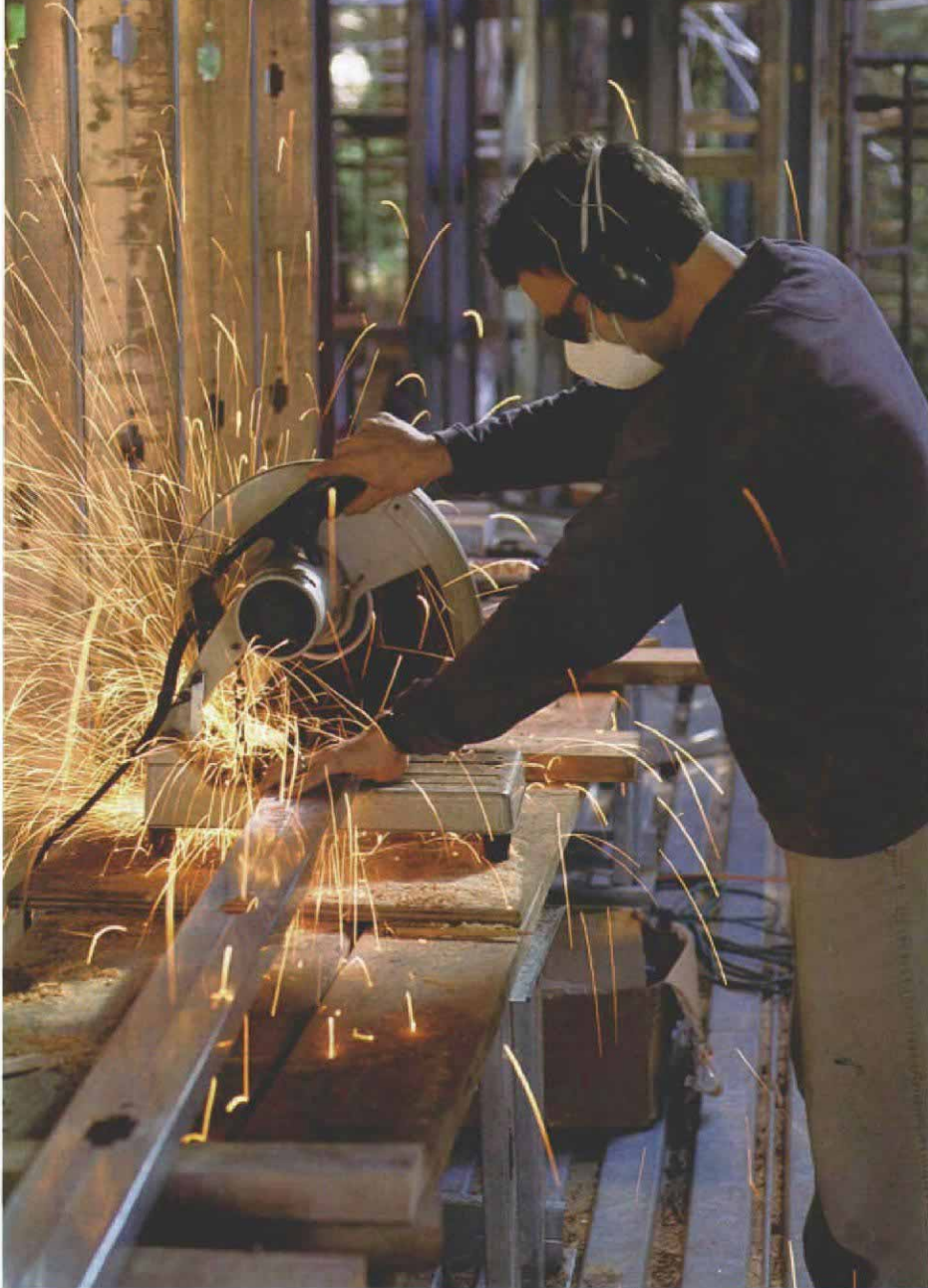
Take the studs to the saw. A cut-off saw with a composition blade is the standard method of cutting steel-framing components. Cutting sheet metal this way demands adequate safety protection.
