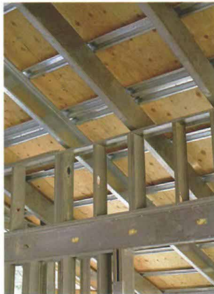
Purlins anchor the roof deck. Purlins made of steel hat channel run parallel with the ridge on 24-in. centers to make a regular layout for affixing the plywood decking to the roof.
