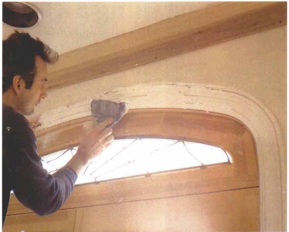
A second layer is smeared on top. A loose mix is spread over the first layer of wet plaster. As the template is drawn over the molding, the loose plaster is forced into the voids left from the initial shaping to complete the profile of the trim.
