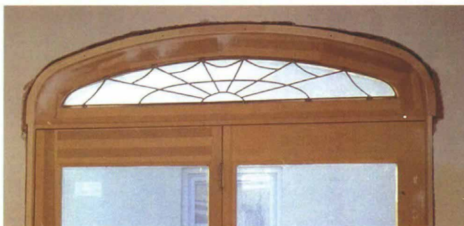
A keyway locks the molding in place. The wallboard has been cut back from the doorjamb, creating a void that fills with plaster and keeps the molding securely anchored.
