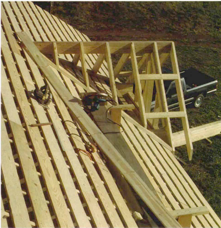
One roof framed on another. A California roof features valley boards that lie flat on the main roof sheathing. As opposed to a valley rafter, there's only one set of jack rafters to cut and one cheek-cut setting on the circular saw.
