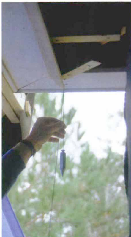
Setting reference lines. The author's system for ensuring flat, plumb walls starts with reference lines hung at the top two corners of the wall. The trim piece just below the soffit is installed so that its inside edge is 8 in. from the sheathing. A plumb line is dropped to the foundation from this point to mark the corner.
