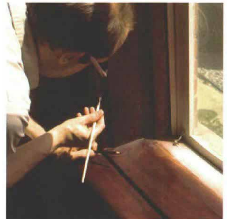
Matching filled areas. Nail holes, cracks and other defects that have been filled must be touched up so that they match the finish.
