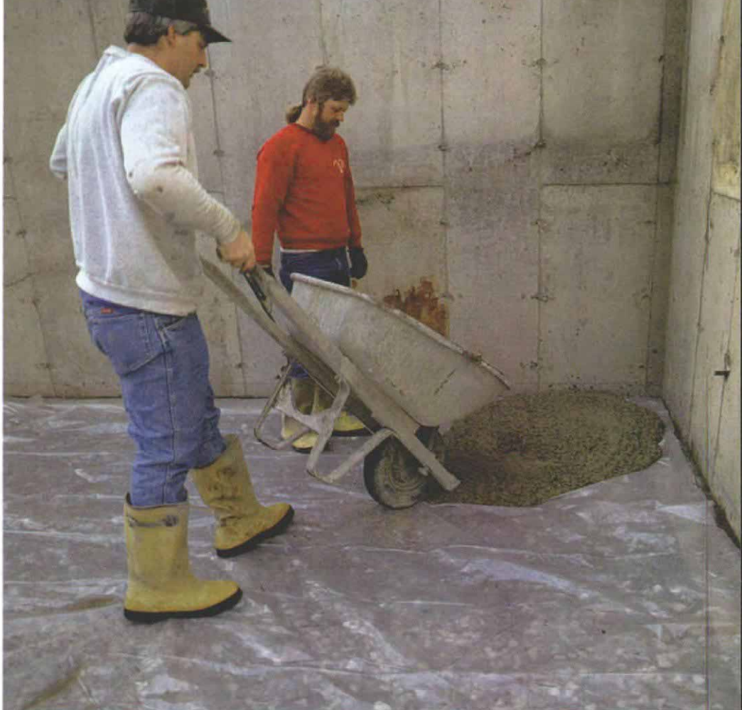
First mud. With the vapor barrier in place and the chalklines snapped, the first load of concrete is dumped in the far corner of the foundation. The mason dumps the concrete away from the wall so that he won't cover the chalkline.
