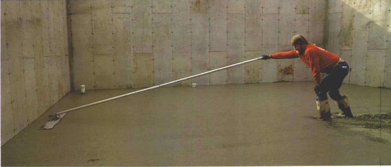
Operating a bull float. After the concrete is screeded, a bull float pushes stones down and brings up the fines—sand and cement—that make a smooth, finished surface. To use a bull float, lower its handle as you push it away, and lift the handle as you pull it back.
