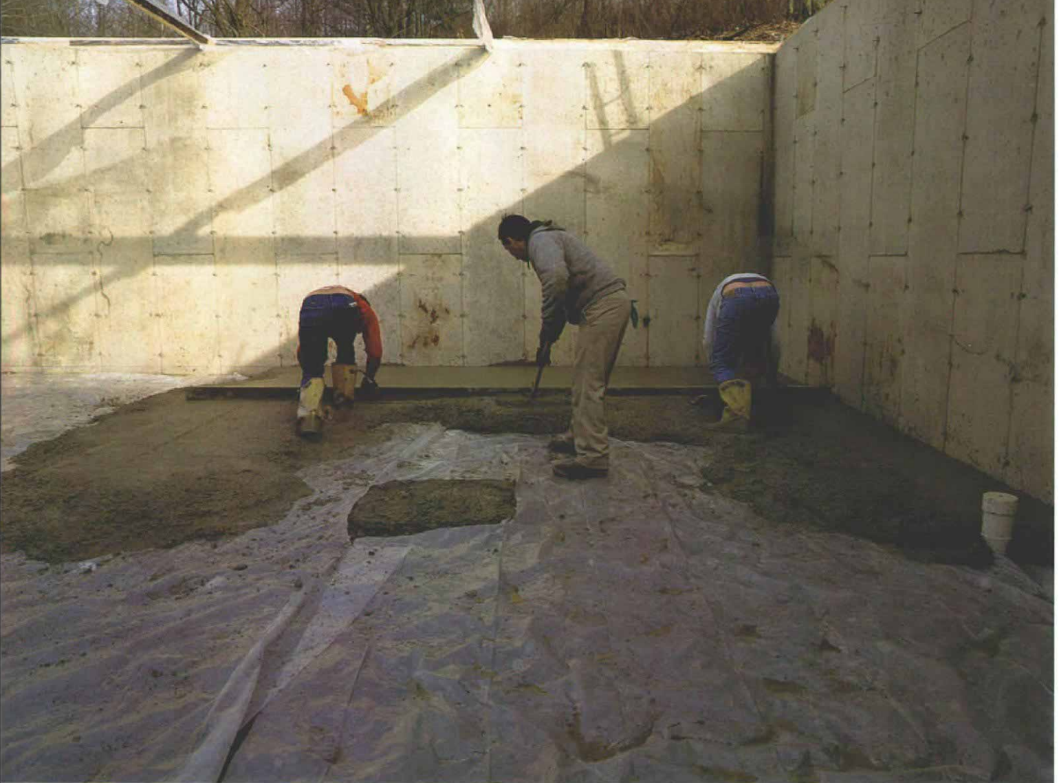
Raker's role. As the screed rail levels concrete between the perimeter screed (right) and the center screed (left), the raker pulls away excess concrete or fills low spots. A rebar spike set at finish-floor height and subsequently driven below the concrete's surface establishes the center screed's level.
