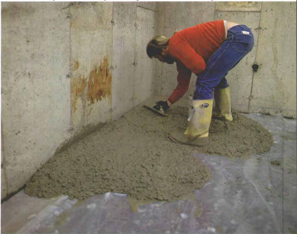
Establishing a perimeter screed. A magnesium hand float is used to push the concrete up to the chalkline. This strip of wet concrete, placed along the foundation walls, is a perimeter screed.
