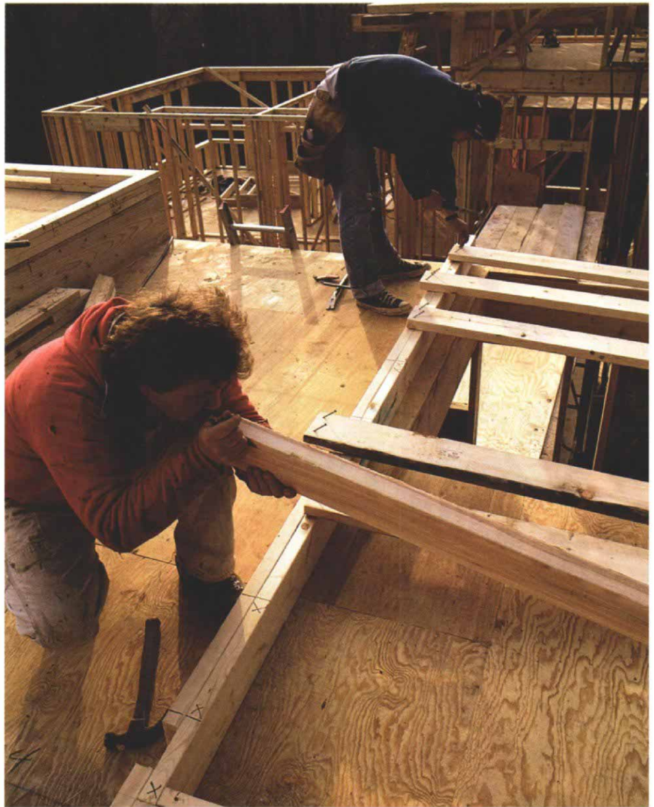
Crowning and toenailing. Sighting down each stud determines its crown. All the studs are then laid on the top plates with the crowns facing the same direction. The toenails are then started in all the studs and nailed all at once, production-line style.
