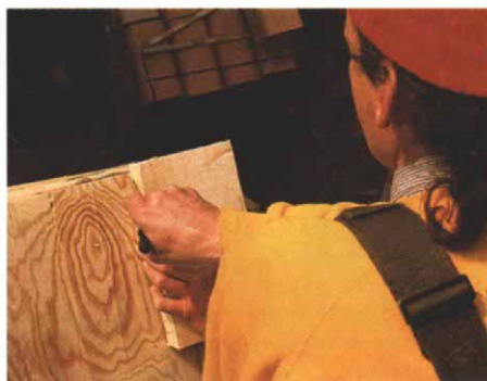
2x6 template. A 2x6 block is used to mark an exterior wall's width on the plywood deck. The author sights down to the floor below to make up for possible irregularities in the alignment of the floor joists.
