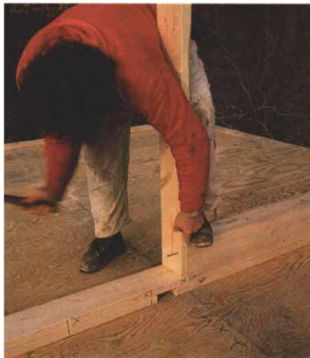
Headers and king studs. Tipping the nailed-together doubler and top plate upside down on the deck makes it easy to toenail the header and attach the king stud.
