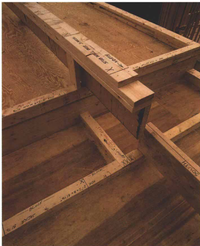
Plated and detailed. Information written on the wall plates and the girders defines how the walls are put together. The author also lays out the second-floor joists or roof rafters before assembling the walls. Different-colored ink is used to denote a change in stud length. (Penciled guidelines were drawn on the lumber only for the sake of neatness in this article. It is not common practice for the author.)
