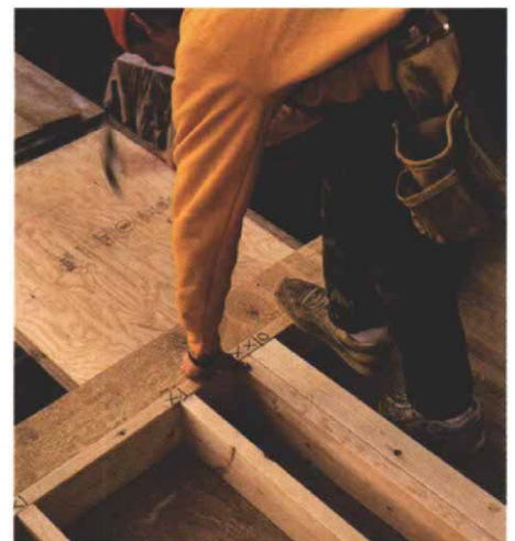
Through-nailing. As in other methods of framing, the author prescribes through-nailing the bottom of the studs, the jacks and the cripples. As he works his way down the plate, he aligns each component to its mark and nails it.
