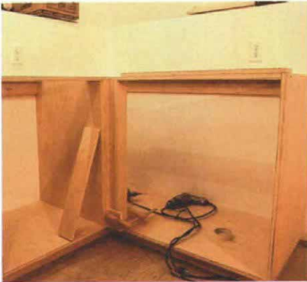
Inside corner. A built-up post made of three strips of plywood serves as an anchor for the cabinet-door hinges. The post is secured at the top by screws through the stretchers and at the other end by a couple of finish nails into the cabinet bottom.
