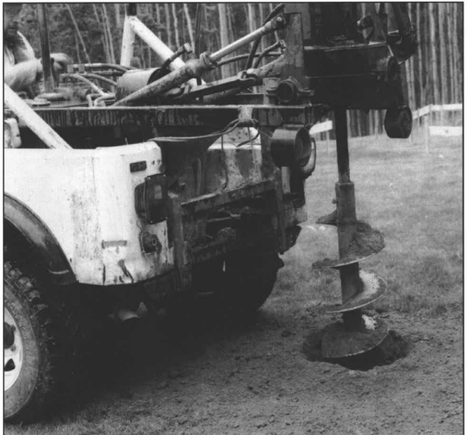
Digging the holes. Holes can be dug in several ways. The author paid the owner of a chain-link fence company to bring in this Jeep-mounted rig. It made short work of a backbreaking job.
