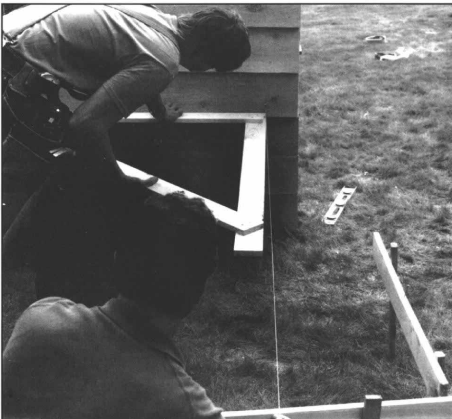
Checking for square. In setting the string to find the corners of the deck foundation, a big, site-built square can be helpful. One leg of the square is held against the ledger board on the house, and the other acts as a reference for attaching the string to the batter board.
