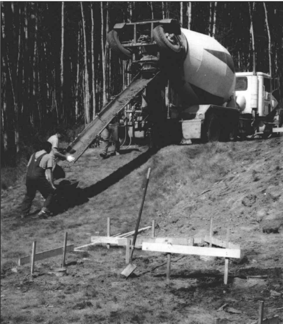
Concrete the fast way. Ordering ready-mix concrete may cost a little more, but it saves a lot of work. Here, a wheelbarrow is used to ferry concrete to the forms.
