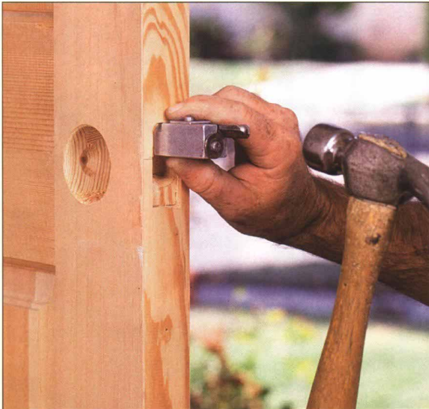
18. Set the corner chisel in the mortise and strike the retractable plunger blade to square off the rounded corners left by the router.
