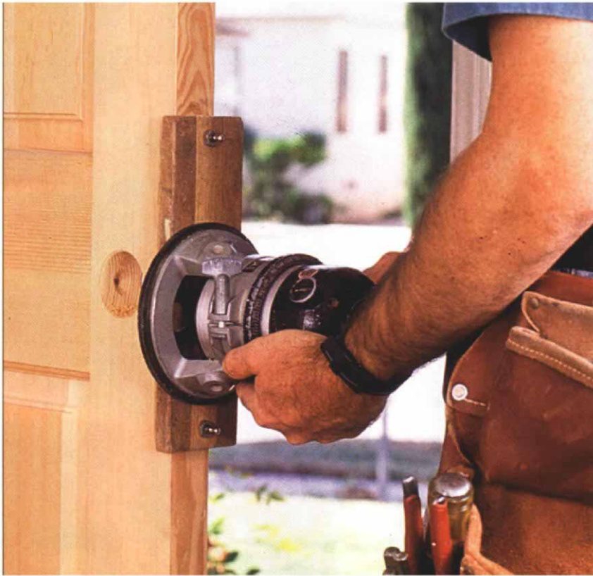
17. A template tacked to the door has an opening that guides a straight router bit set to cut a shallow latch-plate mortise.
