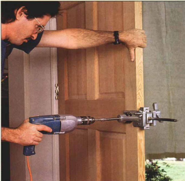
7. Drive the faceboring bit with a drill fitted with a socket adapter.
