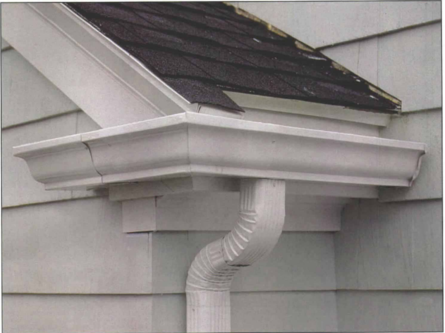
Extending the rake. For a clean look, the top edge of the rake's crown molding extends down past the edge of the roof, where it nearly meets the corner of the gutter. The crown is protected by a tongue of asphalt roofing over a flap of aluminum flashing.
