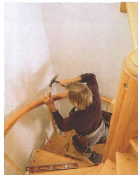
Pass-through balusters. The leading baluster on each tread passes through a mortise to engage the tread below it. White used a 1-in. chisel to square the mortises.
