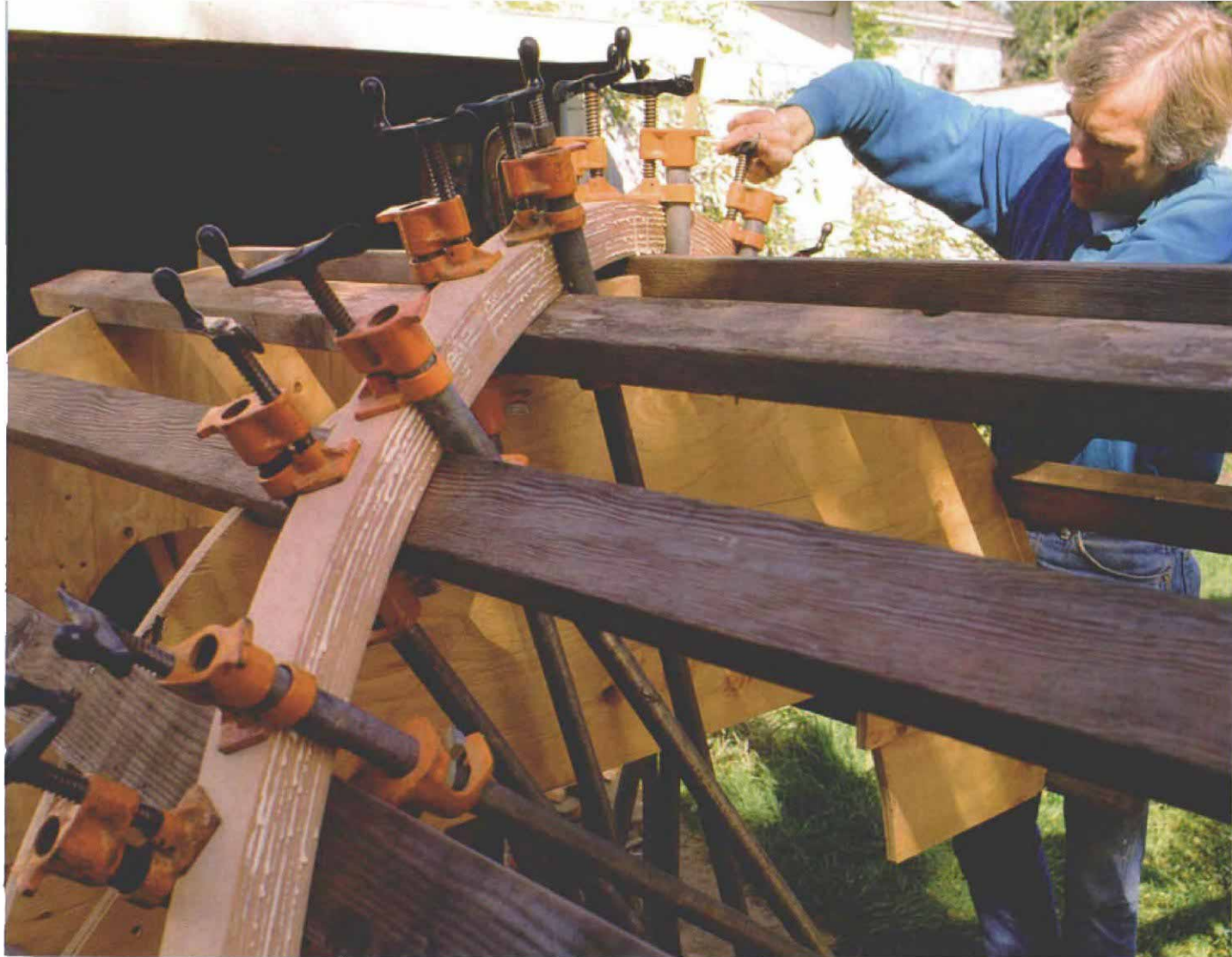
Doing the twist. Stretched across a bending form made of 2x4s on plywood bulkheads that duplicate the radius of the stair, thin laminations of Douglas fir are clamped and glued into a handrail blank.
