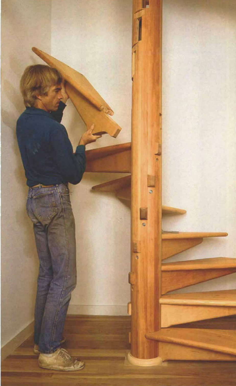
The fan part. Once the column has been slipped over its base and tethered to the landing, White can insert the numbered treads into their mortises, and the stair quickly takes shape. Note the dados above the mortises at the top of the column. The dados accept the ends of the treads, making a clean joint and reducing wiggle.
