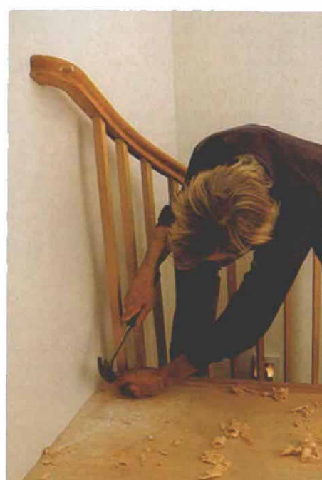
Rail return. At the landing, the handrail engages the wall by way of a curved section cut from a solid piece of stock. Its bolt hole is plugged with a dowel.
