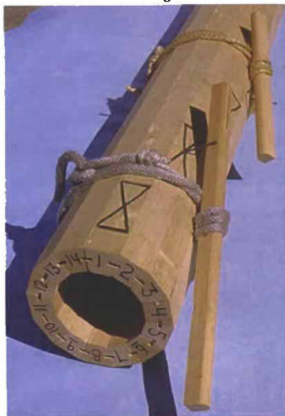
Column glue-up. Subassemblies of glued-up staves are clamped together so that their bottoms are in alignment.
