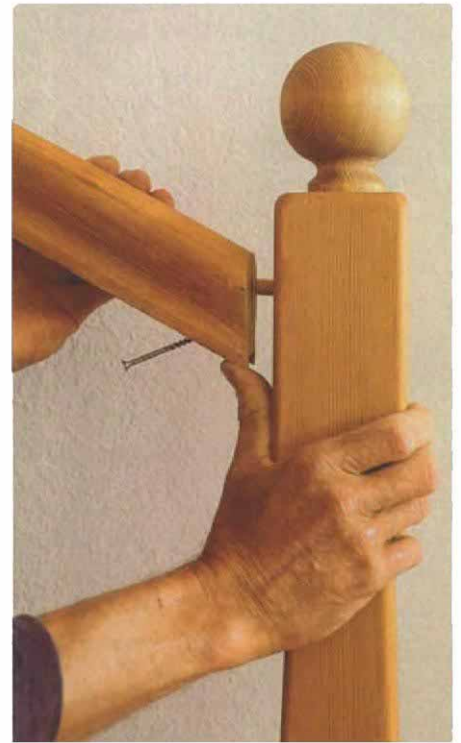
Rail-to-newel. At the starting newel, the handrail is affixed with a \frac{1}{2} -in. dowel and a 2-in. galvanized drywall screw.
