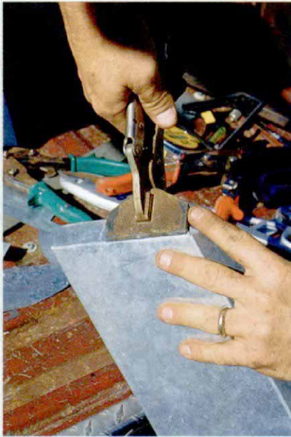
A mitered corner on a fascia gutter is attached by tabs on the end of one of the gutters. Here Williams uses a pair of hand seamers to bend back the solder tabs.
