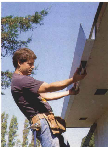
A fascia gutter is a simple U-shaped channel with a flat face that tilts outward. Here the author checks a section for positive drainage toward the outlet.
