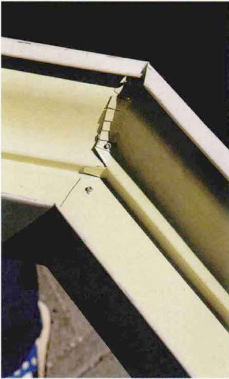
Mitered angles that don't fit off-the-shelf miter strips are reinforced with tabs and rivets. Note how each tab has been formed by removing V-shaped sections on either side. At the gutter's contours, the point of the "V" corresponds to the inside and outside corners.
