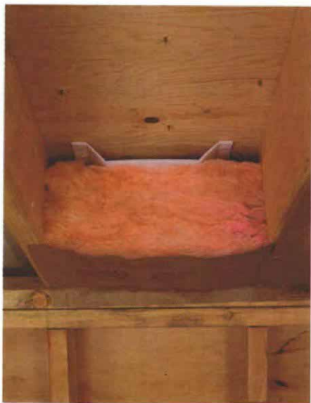
The most common way to vent a cathedral ceiling is with polystyrene baffles stapled against the roof sheathing to prevent the fiberglass batts from blocking the air path in the rafter bay.
